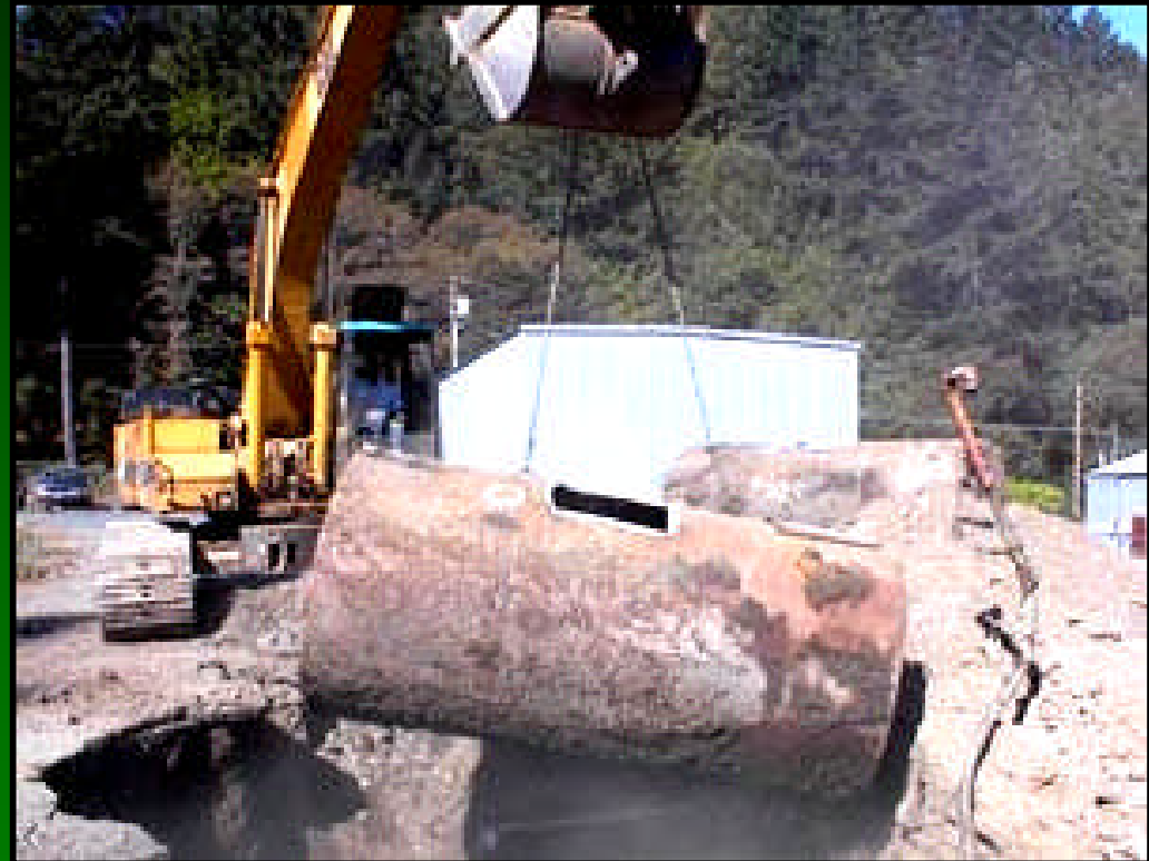
Excavating a leaking UST (LUST) and preparing the cavity for soil sampling.
